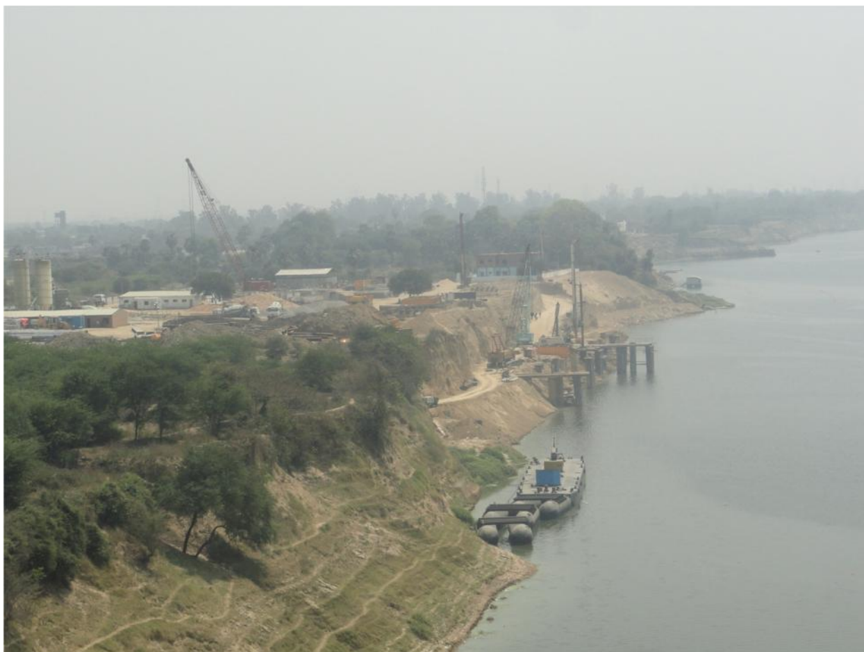
Figure 18: The Ramnagar terminal of National Waterway 1 under construction in Varanasi on the banks of River Ganga.
