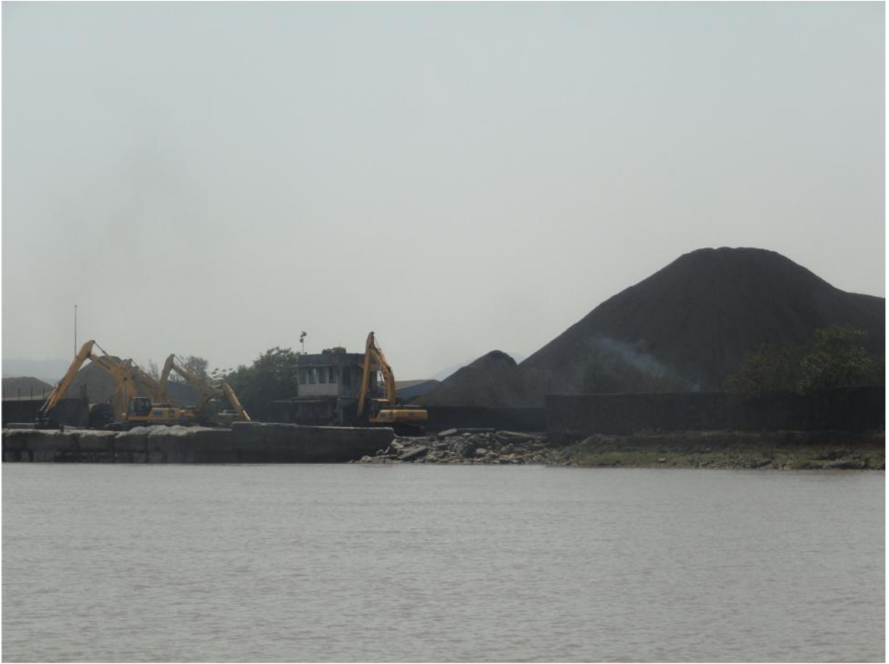
Figure 16: Excavator in operation at jetty of Dharamtar port. Coal stock is seen in the background.
